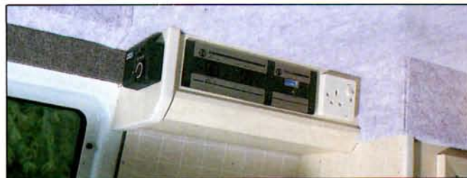
Zig SP4 12v electrical control panel and fresh water level gauge; adjacent mains socket is positioned over worktop area
