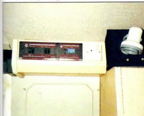
The Zig units show the battery condition and the water level. The spotlight is good for night-time reading.
